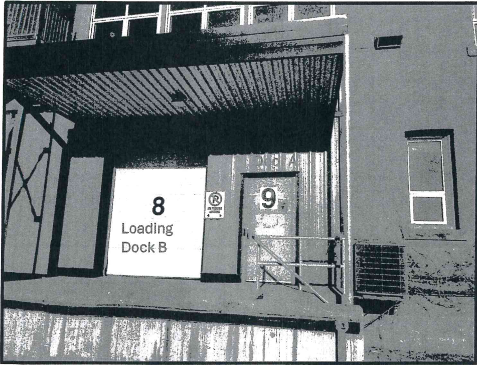
Photo 2: Dropoff Door A and Loading Dock B as per the Site Map in Photo 1.
